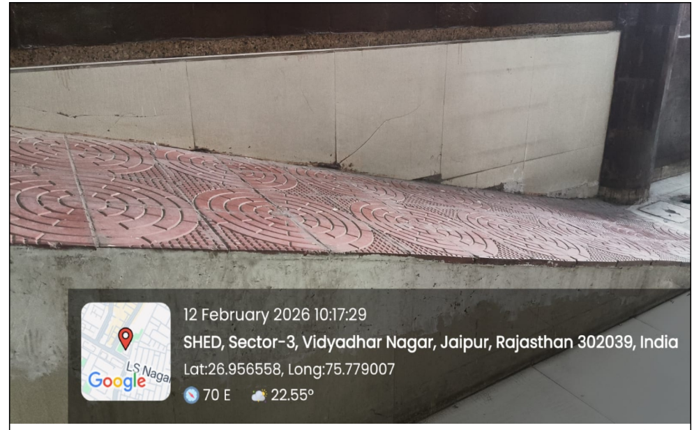
RAMP LEFT REAR
